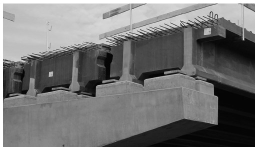
Figure 2. Road bridge at Bourg-les-Valences (France). Central pier during placing of \pi -shaped beams.
